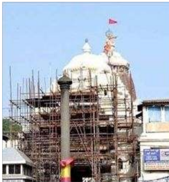
Figure 3: Repair of the Jagamohana (audience hall) of the temple (Source: Odisha Sun Times)
