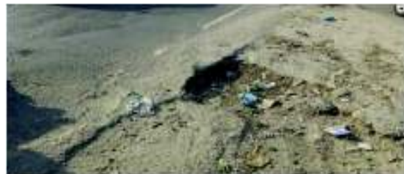
Figure 8: Edge cracking and shoulder drop off
