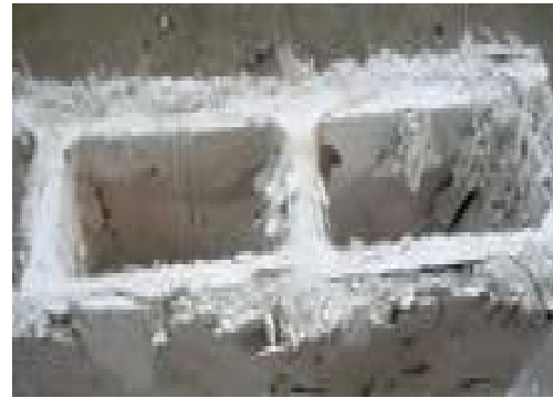
Fig. 2 Crack in the Empty GFRG Panel
