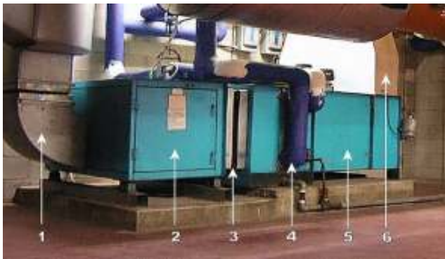
Figure 7: An Air handling unit is used for the heating and cooling of air in a central location
